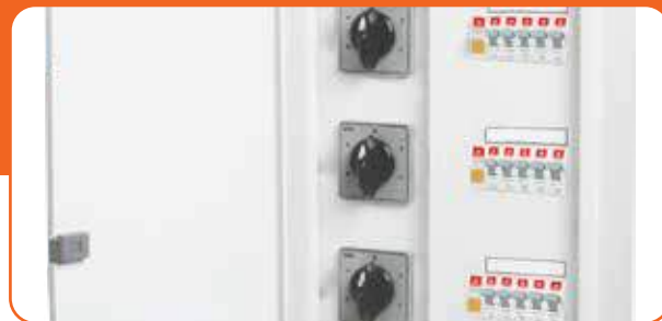
Manual phase selector DB which allows shifting to healthy phase using phase selector switches
